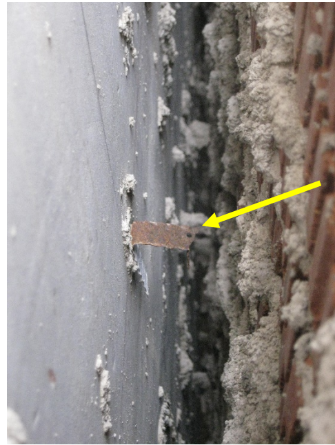
Figure 14. Corroded and failed veneer anchor at a portion of the wall that had not yet collapsed.
