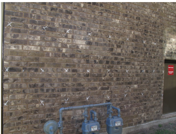
Figure 8: Overview of typical survey area at brick masonry veneer (anchors denoted with chalk "x" markings).
