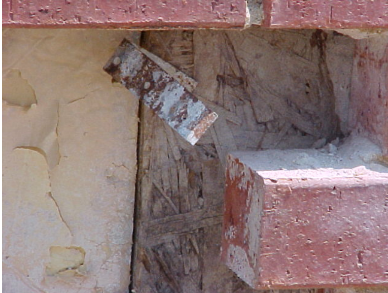
Figure 15. Veneer anchor corrosion at a structure less than one-year of age.
