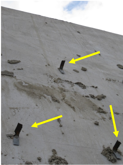
Figure 13. Corroded and failed veneer anchors at a collapsed veneer wall.
